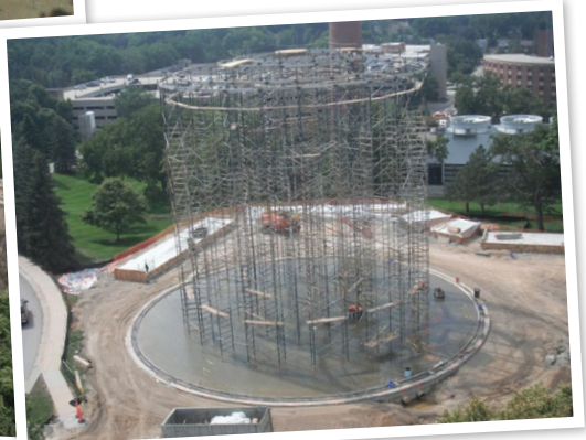
Scaffolding in place to support construction of center portion of concrete dome.
